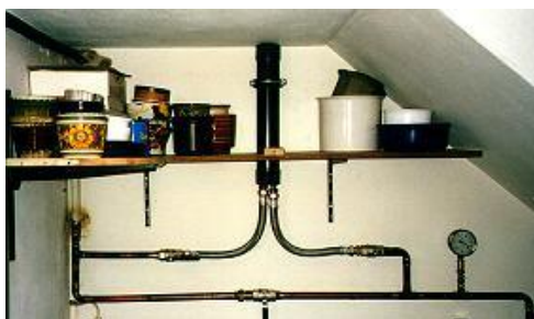
Installation after the water meter.
